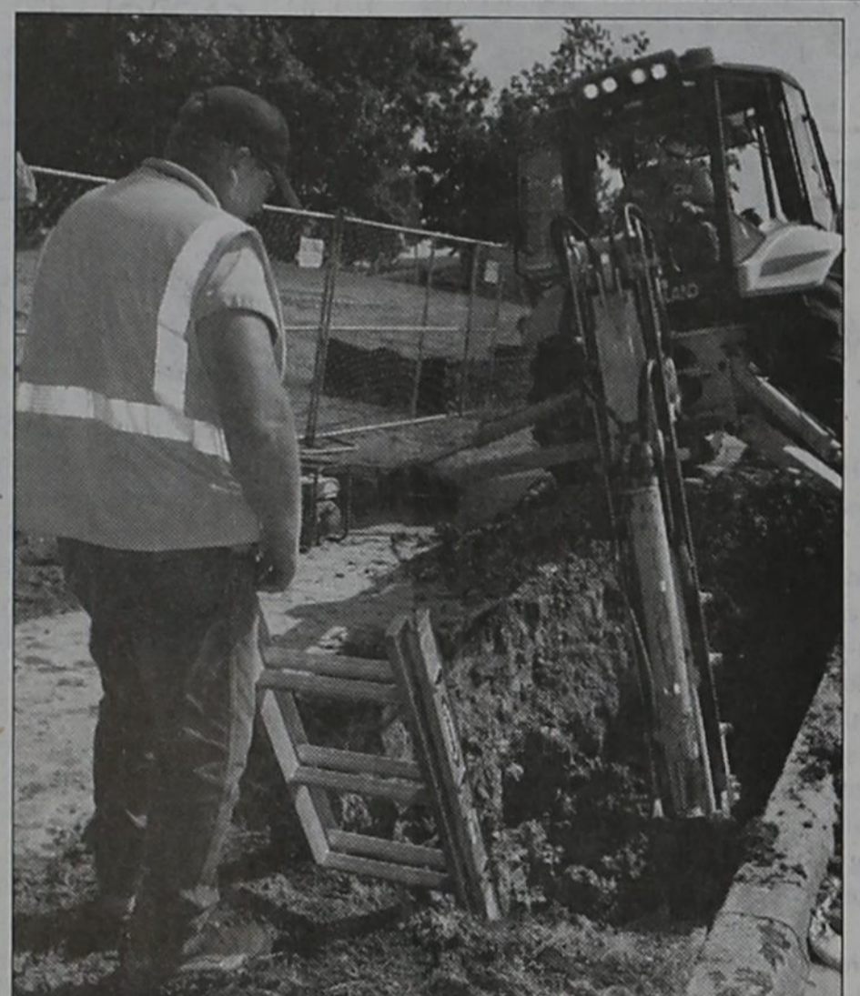
City of Rockwall Water Department Field Supervisor Curtis McAden (left) watches as Johnny Seals (right) operates the backhoe while repairing a broken water supply line on Thursday, July 17 on Yellowjacket Lane. Staff photo by Tim Burnett
