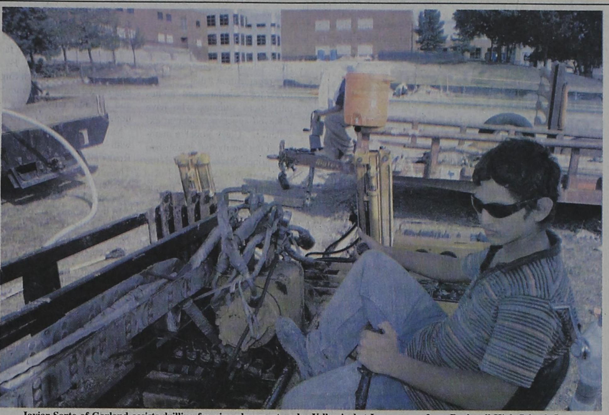
Javiar Sorto of Garland assists drilling for pipe placement under Yellowjacket Lane across from Rockwall High School. Sorto works for JMR Brothers, Inc. also of Garland. Staff photo by Tim Burnett
