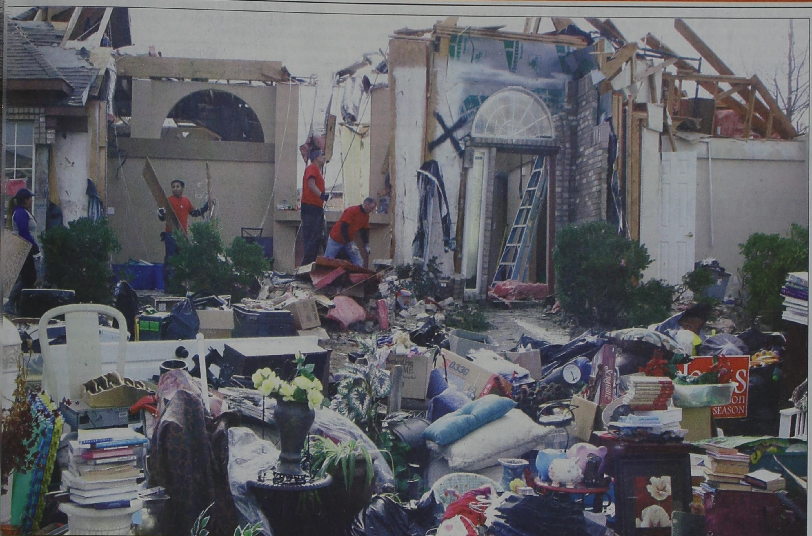
A team of volunteers with Operation Elevation (wearing red shirts) assist in clean-up efforts, Tuesday Dec. 29, 2015, at the intersection of Linda Vista Drive and Luna Drive (just west of Dalrock Road) in Rowlett, following the Sat. Dec. 26 tornadoes that destroyed many homes in Garland and Rowlett. Under the direction of Elevate Life Church in Frisco, Texas, the team arrived on the scene, Sun. Dec. 27, and began to assist the home-owners. According to the church's website, another team will arrive later in the week to assist in clean-up and serve where needed. Photo by Tim Burnett/Rockwall County News
