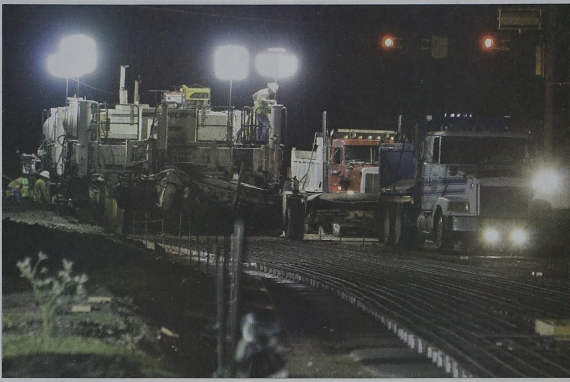
Overnight road construction on FM 740 (Ridge Road) and Summer Lee Drive continued Monday evening in Rockwall. Progress is being made, but curb inlets, manholes and the numerous driveways required to adequately accommodate homeowners' access have slowed paving operations somewhat, according to Texas Department of Transportation project manager Kerry Lively. The second pass of paving should go more quickly. Pending weather conditions and the continued cooperation of machinery, the project should be finished the week of Sept. 6 after the holiday weekend.
