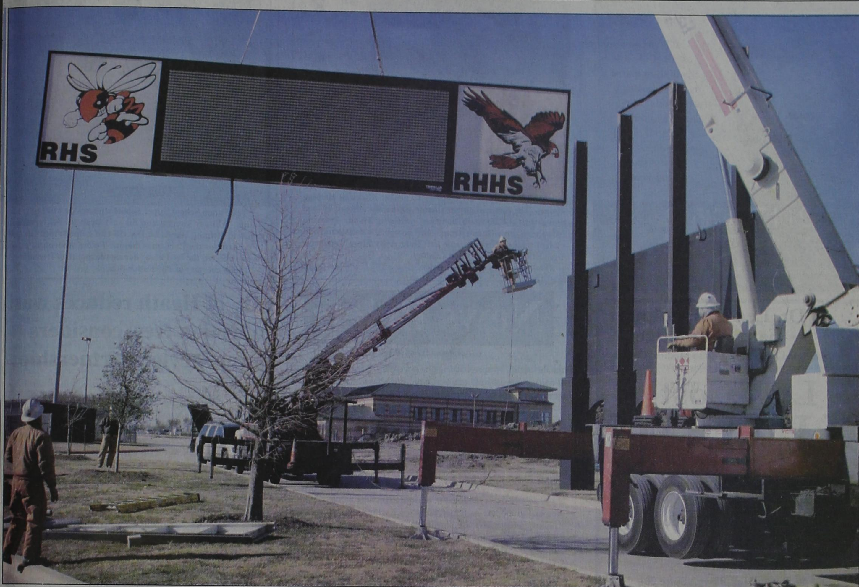
The final monument for the old Wilkerson-Sanders stadium in Rockwall came down Wednesday, January 15 when the scoreboard was removed as part of a major renovation project. The scoreboard was installed in 2000 by Daktronics, recording the victories and defeats of local
