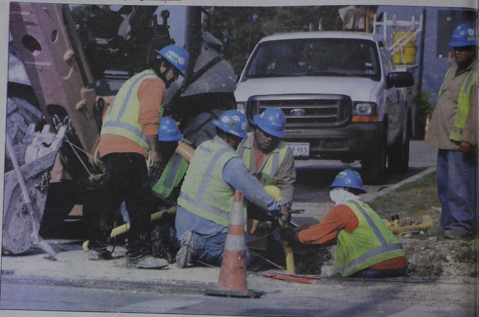
TxDot workers dig their way through Washington and Goliad in downtown Rockwall in preparation for future street improvements of the 205/Goliad street expansion project that north from I-30 towards downtown. Staff photo by Tim Burnett
