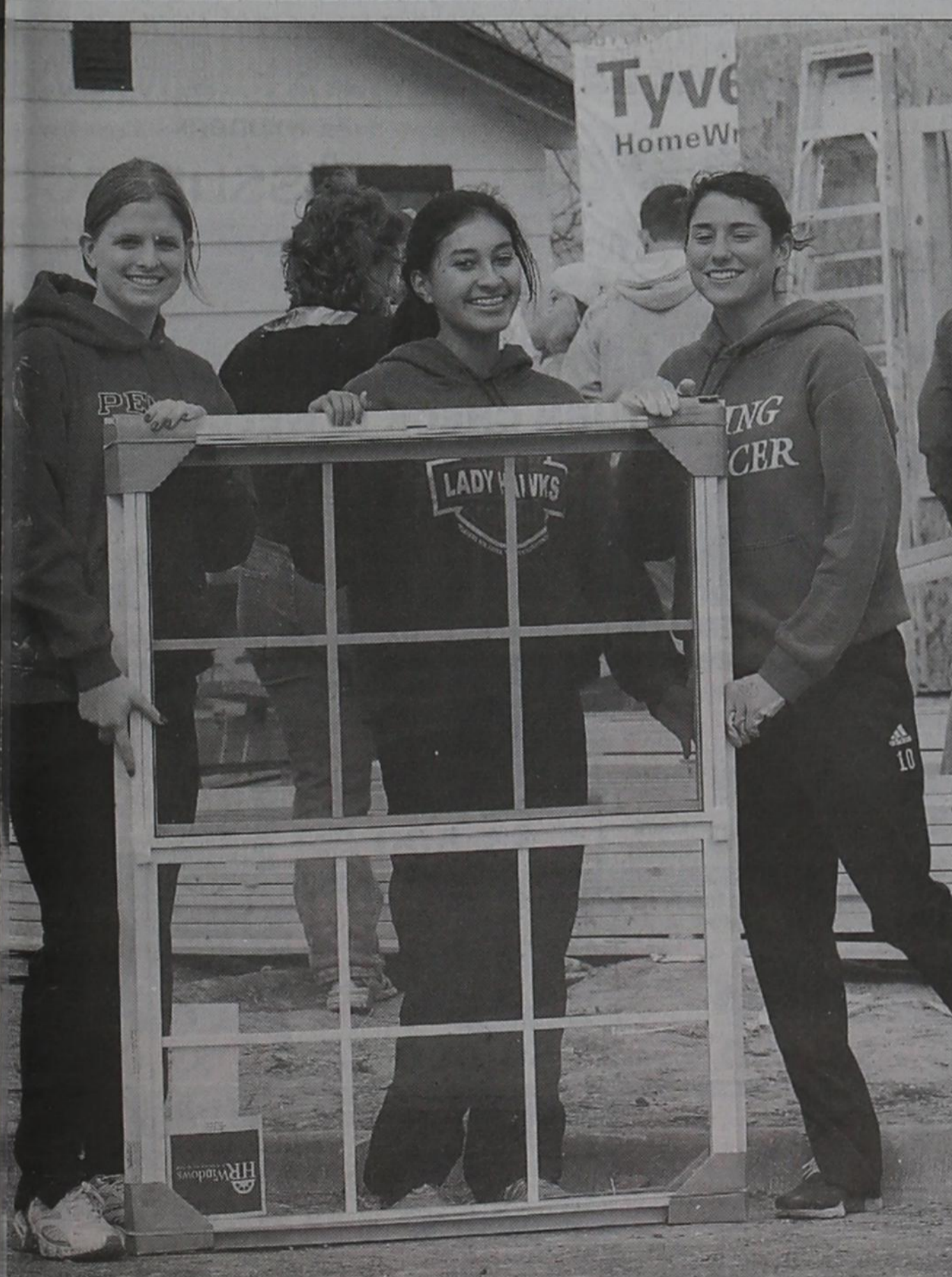
Krista Heinrich, Cassie Munoz and Vanessa Boice (left to right) move windows and other supplies as they volunteer at the latest Habitat for Humanity home building site in Roysse city. The house is expected to be completed in about five months and will be owned by Deidra Culp and her children, Sarah, Sophia and Seth.
