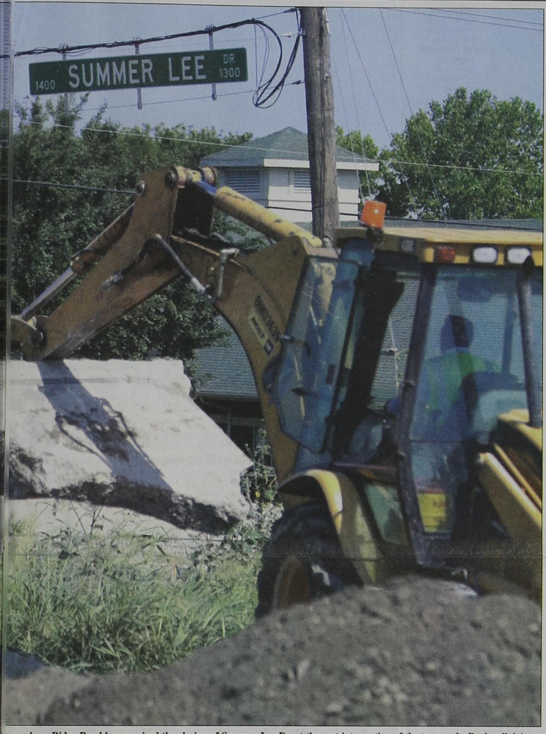
Work on Ridge Road has required the closing of Summer Lee Dr. at the east intersection of the two roads. Rockwall drivers, along with the construction bottle-necks, are easing through the maze with courteous and considerate behavior. The Summer Lee Dr. and Ridge Road intersection is expected to be open on or about July 15.
