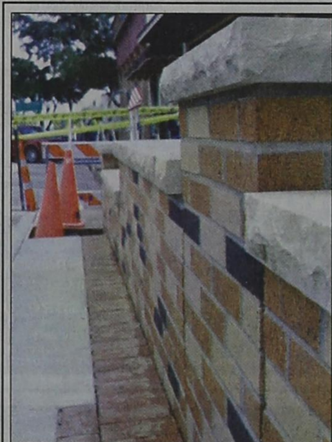
On Monday, September 15, the Rockwall City Council voted to keep the current modern pattern on the renovation of the downtown square.
