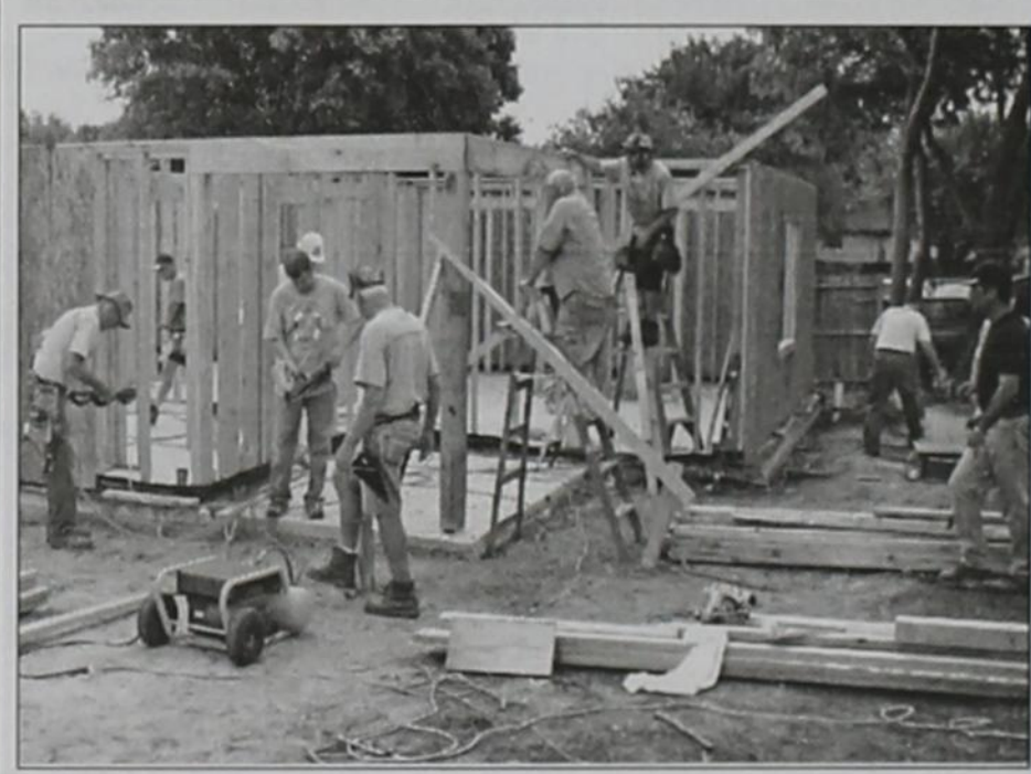
Work continues for the fourth week on Peter's Colony Drive in Rockwall on the latest house by Habitat for Humanity Rockwall Area. The three-bedroom, two bath home will be finished in 20 to 26 weeks, depending on the weather as fall sets in. The walls are up and this weekend, workers are expected to raise the roof trusses. Working on the porch supports were (back on ladder) volunteers Gabriel Bennett and (front) Larry Lazinski. In October, Habitat expects to begin work next door to this house on a fully handicapped accessible home. To volunteer or donate a meal to workers, visit www.rockwallhabitat.org .
