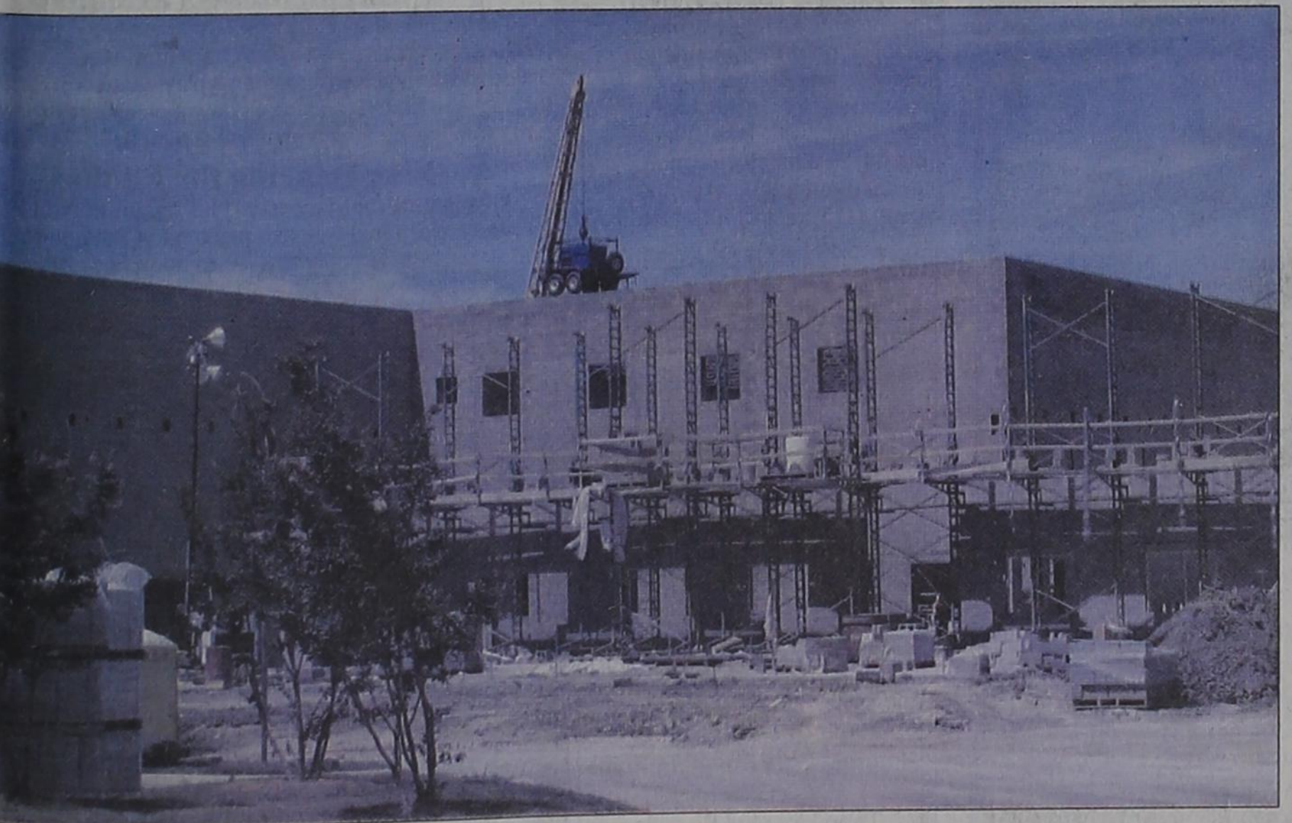
Expansion has begun at Rockwall Heath High School. The new fine arts wing will house a 3-tier, 1,500-seat performance hall, new band practice rooms for orchestra and choir, and make-up and dressing rooms. The addition is expected to be ready for the 2010 school year. Photo by Sean Williams
