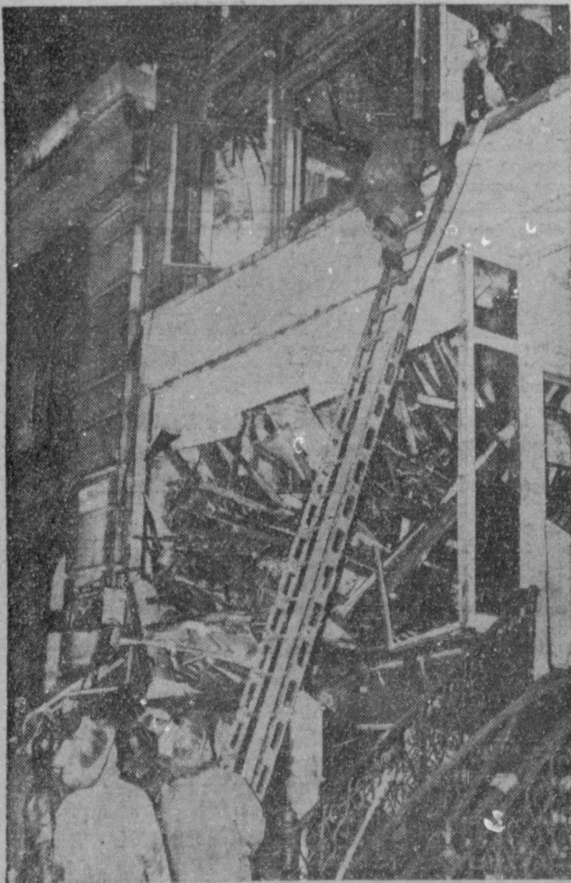
TWO DIED HERE —When fire-weakened upper floors of this New York building collapsed while the flames were being brought under control, two fire insurance company patrolmen were trapped and died where they fell. Here firemen probe the remains of the building for possible unknown victims.
