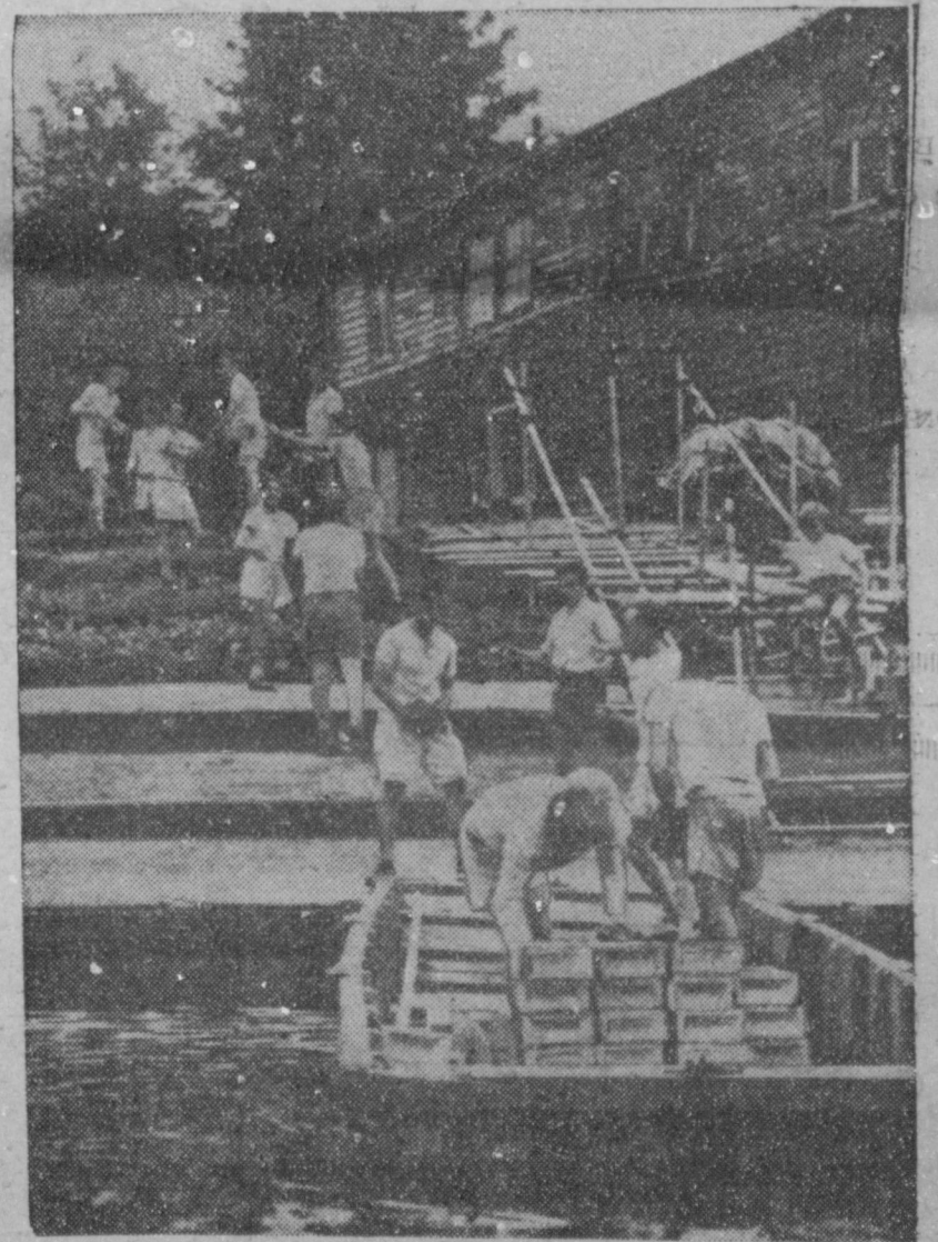
EVERYONE'S IN ON IT —Members of the rowing club in Twickenham, England, decided they needed a new boathouse and the cheapest way was to build it themselves. Here they load brick for transportation to the building site via a brick brigade.
