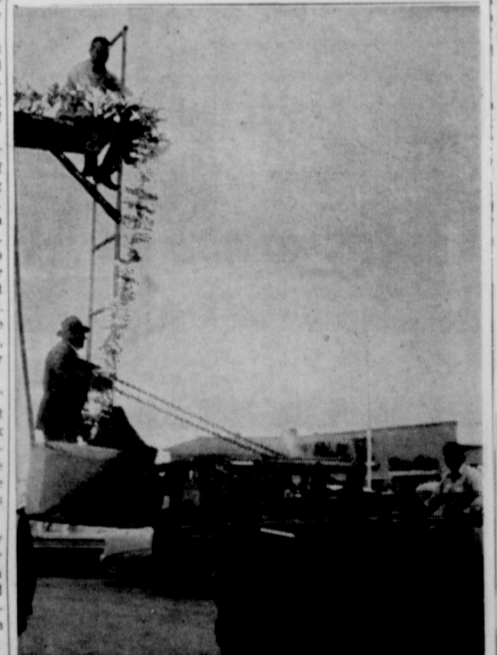
CHRISTMAS TINSEL AND related decorations were installed this week across Slaton streets in preparation for the Saturday visit of Santa. Atop the ladder in the operation pictured above W. L. Hendricks, Ernest Alverado immediately below. Grady Inder, barely got into the scene at left, while tractor operator D. Deane smiles broadly at the Slatonite photographer.
