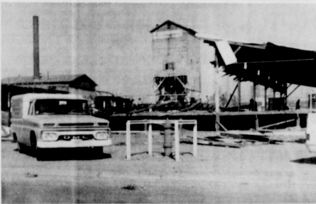
BIG REMODELING JOB — A real "face-lifting" is underway at Union Compress in Slaton where about 16,000 square feet of floor space is being completely rebuilt around the press area, which can be seen standing above the torn-down area in the middle of this photo. (Slatonite Photo)
