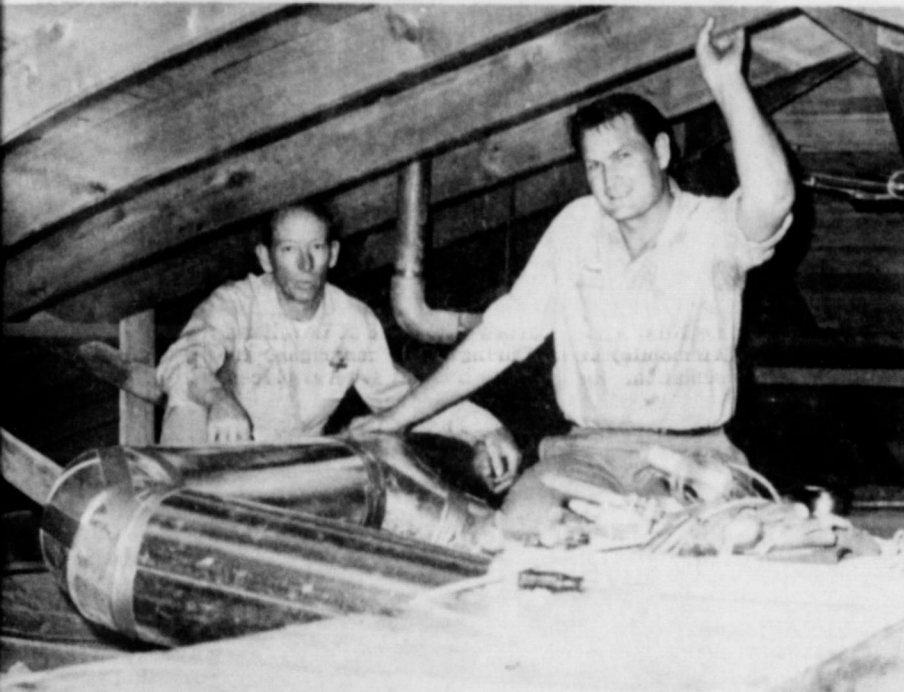
BY THE WEATHER DOCTORS, shown completing duct work in the Edwards' home . . .
