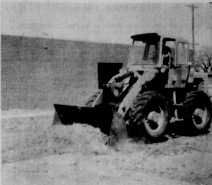
LEVELING PLAYGROUND --Leveling the playground at the Day Care Center at Evans School is this city grader operated by E. D. Duncan, city employee. (SLATONITE PHOTO)
