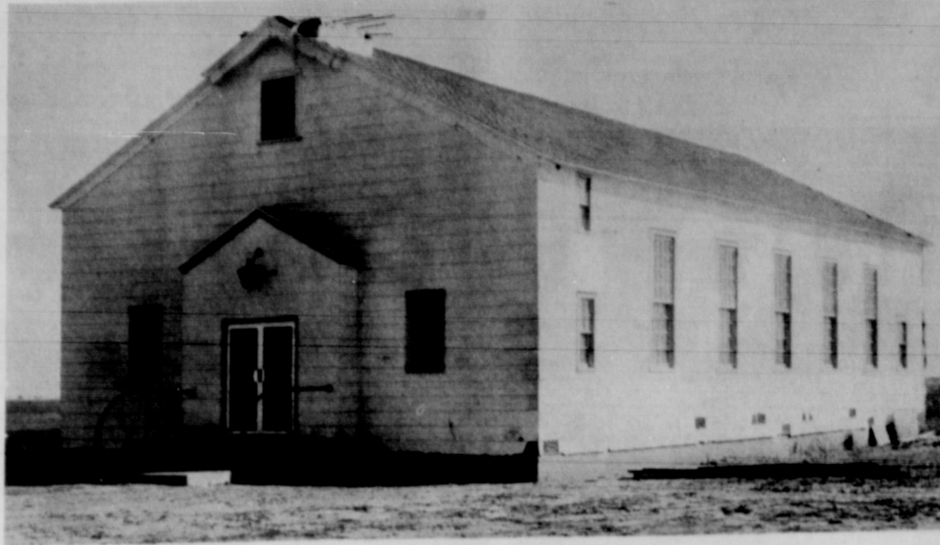
HERE'S THE CHURCH, HERE'S THE STEEPLE -- If all goes well this weekend, workmen hope to get the steeple in place on the old Reese Air Force Base chapel which has been moved to Cooper by the Cooper Church of Christ congregation. The chapel is one of the original buildings built at the air base west of Lubbock. (SLATONITE PHOTO)
