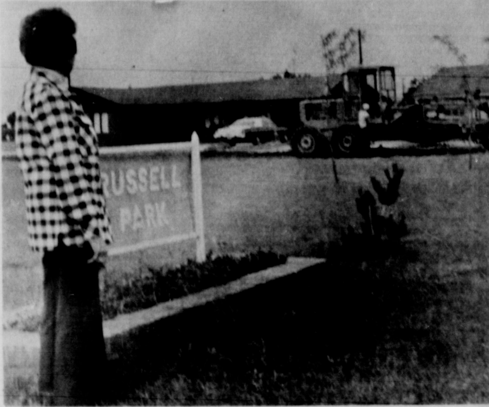
RUSSELL PARK — Mrs. Joe L. Miller is shown watching the paving process now going on at Russell Park. Mrs. Miller donated the land for the park to the city, and the first paving in that addition was done in 1959. When the horseshoe drive into the park is finished, paving for the entire addition will be complete. Lots around the park are for sale. (SLATONITE PHOTO)
