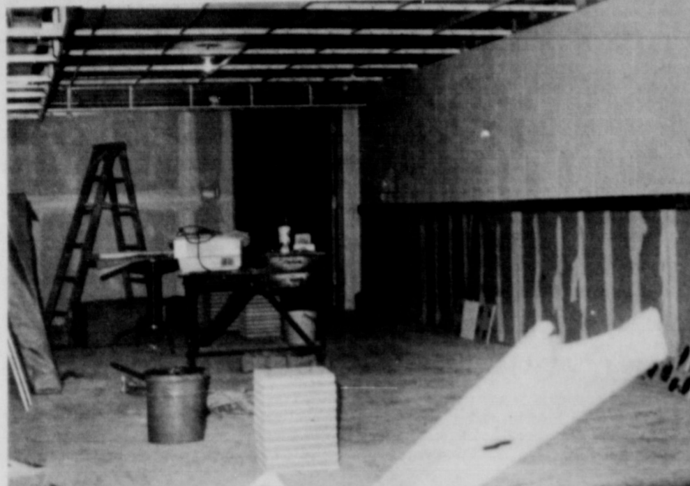
BANK RENOVATION — Work is currently underway in the basement of Citizens State Bank as part of an extensive renovation of the bank building. The basement, which was previously used for storage, is being converted into the bookkeeping department. A drop ceiling is being installed, acoustical tiles are being put up, and carpet eventually will be laid. (SLATONITE PHOTO)
