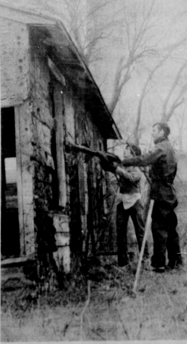
FIRST ONE — This city owned house at 1055 S. 5th was the first one to be demolished in Slaton's cleanup campaign. Skip Crawford and an unidentified co-worker of Slaton Service Co. were in charge of tearing down the building. The work was complete by the end of the afternoon. (SLATONITE PHOTO)
