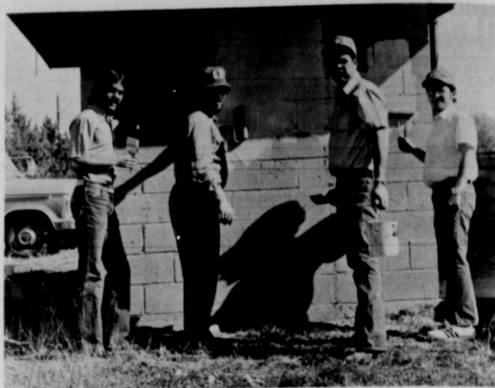
JAYCEE PROJECT — Members of the Greater Slaton Area Jaycees spent Sunday afternoon painting the little league baseball park. Members shown from left are Landy Bowns, Marlin Payne, Jim Dulin and Ted Dawson. The Jaycees decided to repaint the building because earlier in the year someone had written four-letter words on it in silver and gold paint.
