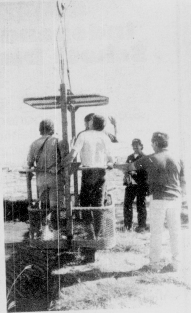
Proud workers and a brave photographer head to the top of the Cross to untie the final guide rope.
