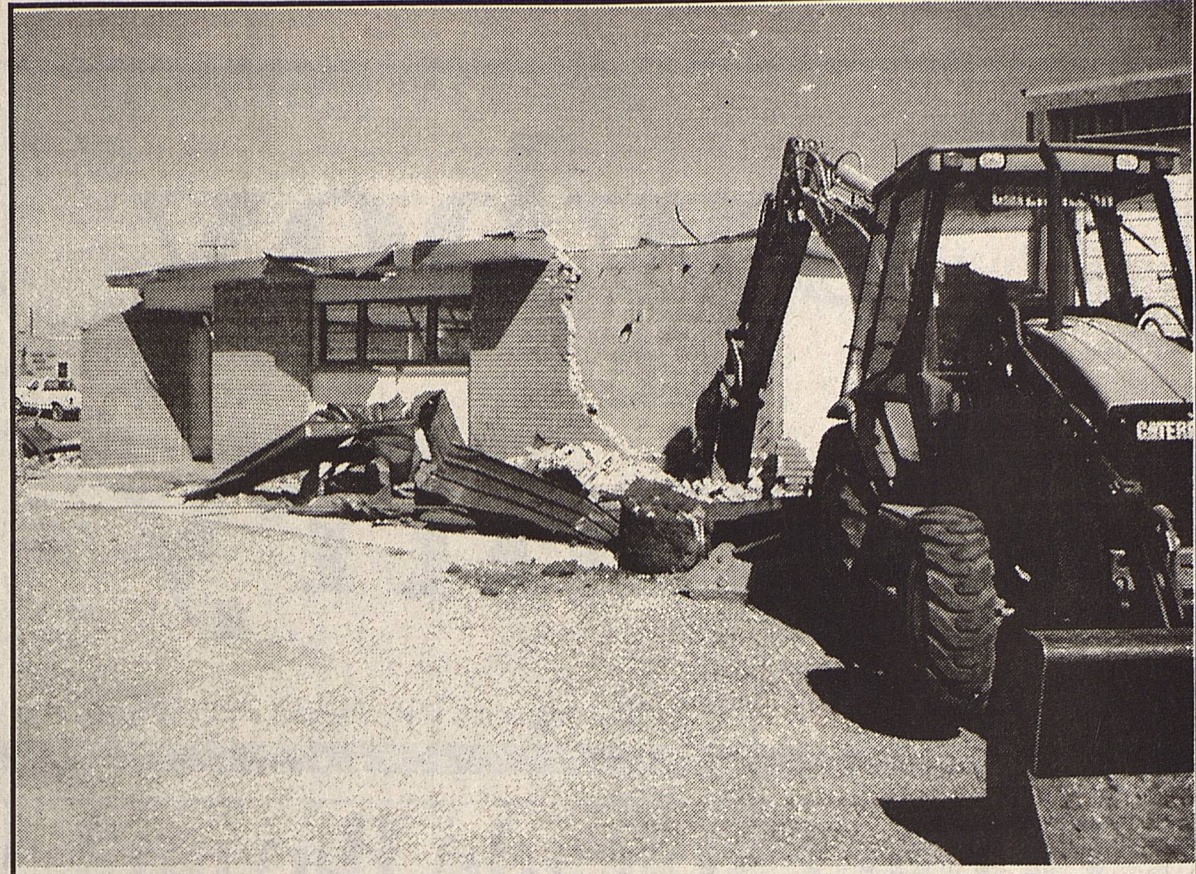
This City backhoe, with help from County loaders and trucks, made short work of demolishing and removing the old City Hall building. Dirt work is now being completed at this site for pouring cement for the new city facility. Actual construction work is scheduled to start soon.
