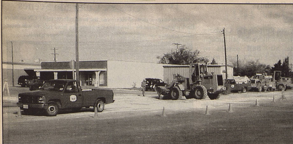
County Pct. 4 employees were busy last week preparing to resurface the street at the northeast corner of the courthouse. A ruptured water main had to be replaced, leading to the resurfacing.
