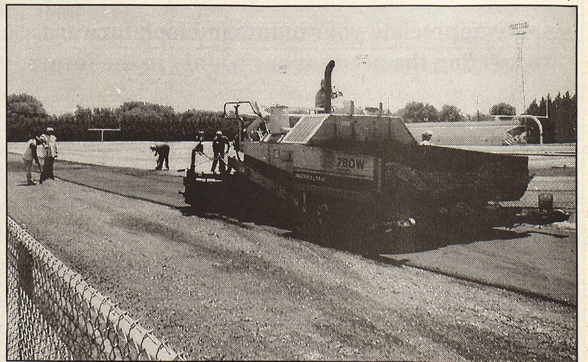
On a recent hundred degree afternoon, this crew was laying a new asphalt base for the running track at PISD. Another contractor will later add the rubberized top coating. The previous track was twenty years old and was deteriorating badly.
