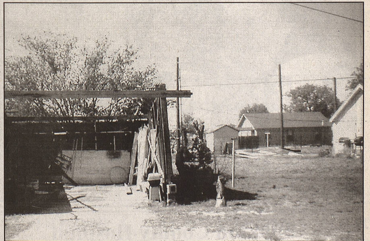
High winds which whipped through town last Thursday night took their toll on shrubs and trees, and the garage/storage building shown here. Sheet iron ripped from the roof of the structure is shown scattered in the right background of the photo. The wind was accompanied by rain reported two-tenths to one half inch in gauges around town.
