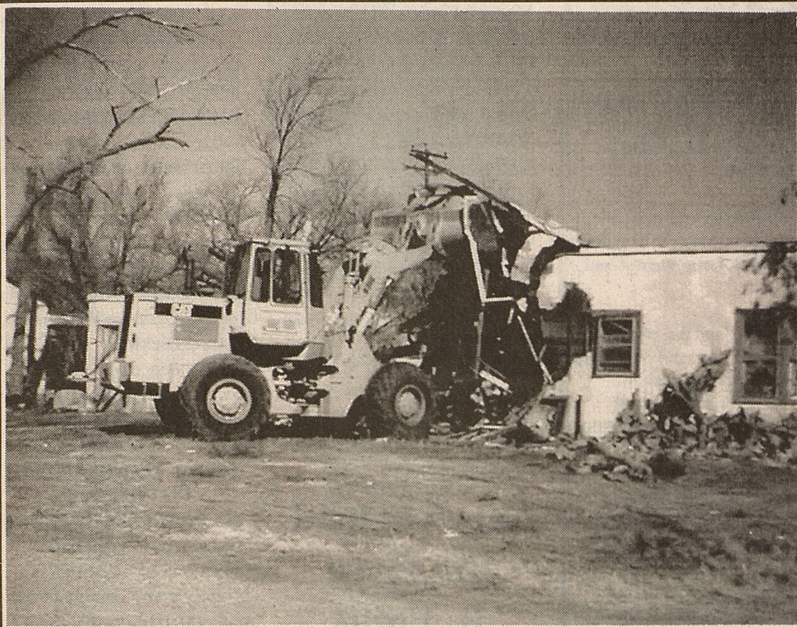
This Pct. 4 Caterpillar loader appeared to be 'eating' this old, empty house on the northwest corner of Moreland and Copeland last week. The County was asked by the city to demolish the structure after it was condemned by health and sanitation officials.
