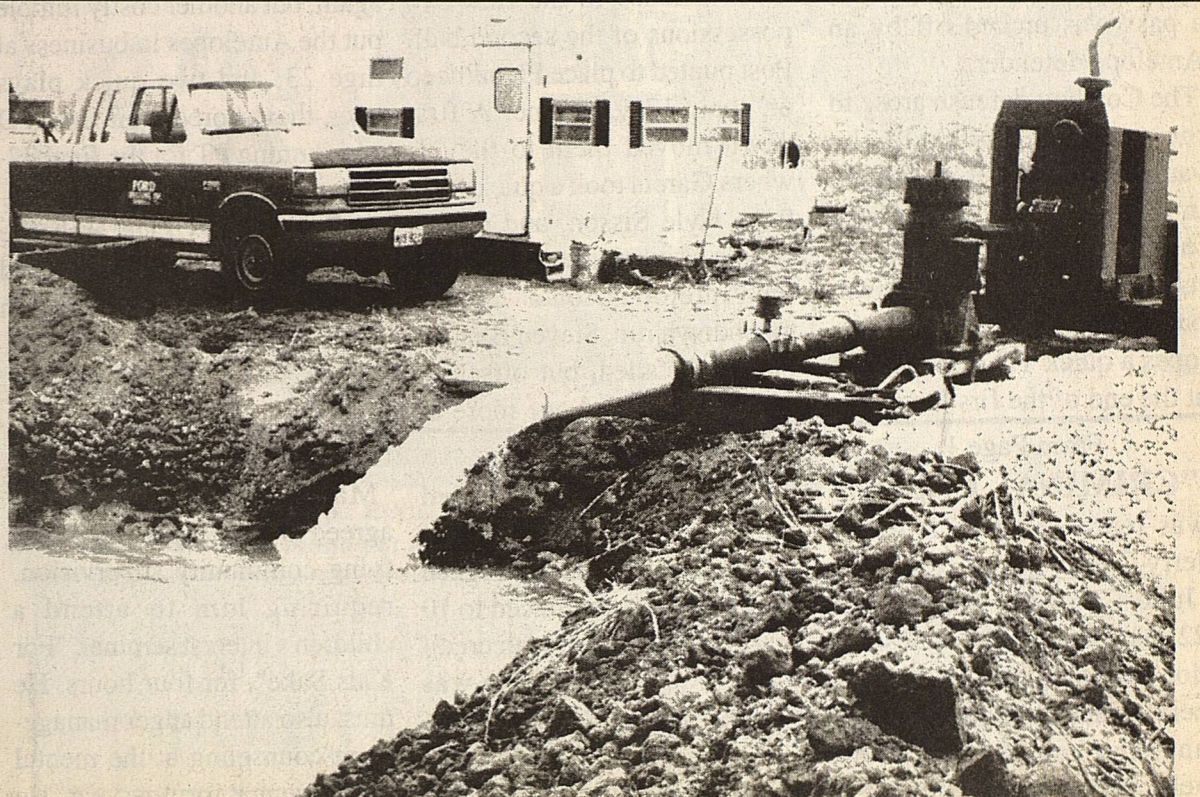
Photo taken last Friday shows new city water well number three on test pump. The flow meter on top of the pipe was reading a discharge of 1170 gallons of water per minute at the time of the photo.
