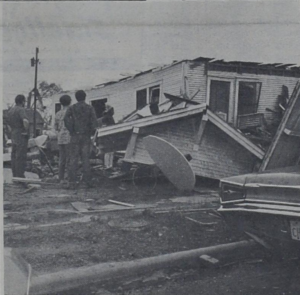
Home Damage in North Lubbock
