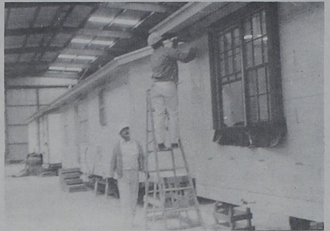
PAINTING STATION —Houses on the assembly line at First Manufactured Homes are mass produced in as little as ten days. At the first station the walls are put up. Later the trim is painted and the interior work is done. (Times Photo)
