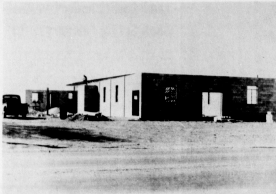
CONSTRUCTION CONTINUES ON CATHOLIC CHURCH, with workmen beginning on the roof following completion of walls and inside room separations. The church is expected to be in readiness for mass within the very near future.
