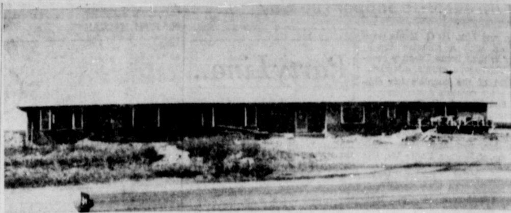
ABOVE is the beautiful new home of Mr. and Mrs. E. C. Clayton, located on the Springlake highway. The 3-bedroom home with den is brick veneer, and has 3225 square feet of space, not including the 24' x 24' 2-car garage. The Clayton's new home has 2 1/2 baths. Construction began about May 15 and will be completed by Sept. 1. (Photo by Taylor Studio, Ltd.)
