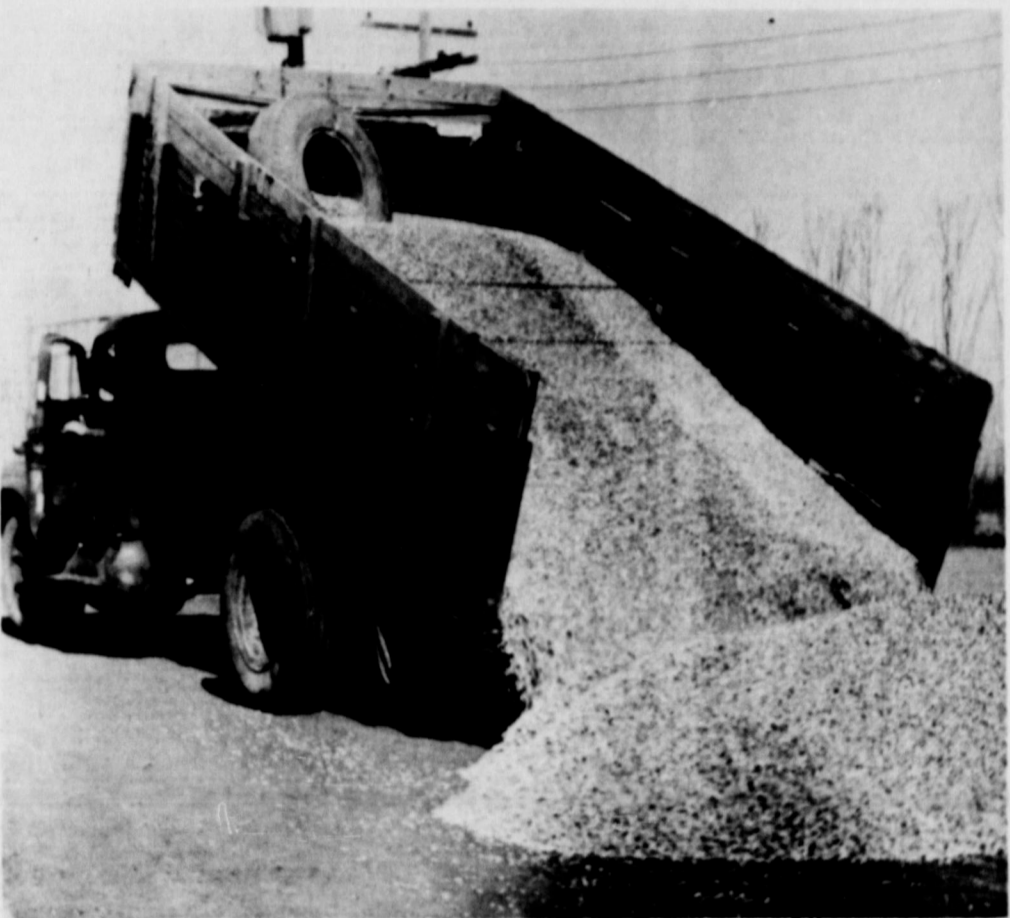
TONS OF NO. 5 ROCK are being unloaded at the Wolverine Stadium to begin the foundation for the new cinder track under construction. Truck shown here is owned by Fred Clayton, and is one of many trucks volunteered by residents to help get the big job completed.
