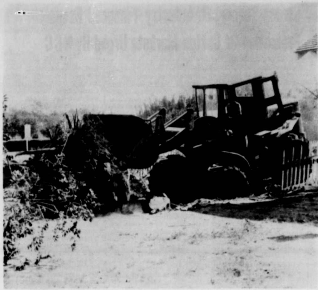
CLEARING THE WAY —Bulldozer removes trees at the future building site of the new Piggly Wiggly supermarket. Fences, shrubbery and trees are cleared away as preparations get underway to move the houses at the corner of Elm and Main.
