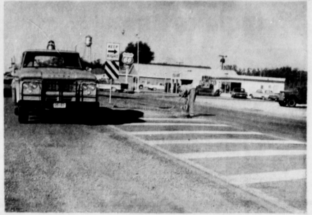
MAIN STREET OF HIGHWAY 70 in the city of Earth took on a new look this week as Highway Department workers, cleaned and repainted the center line. The worker above is shown as he prepares to paint the center line east of town.
