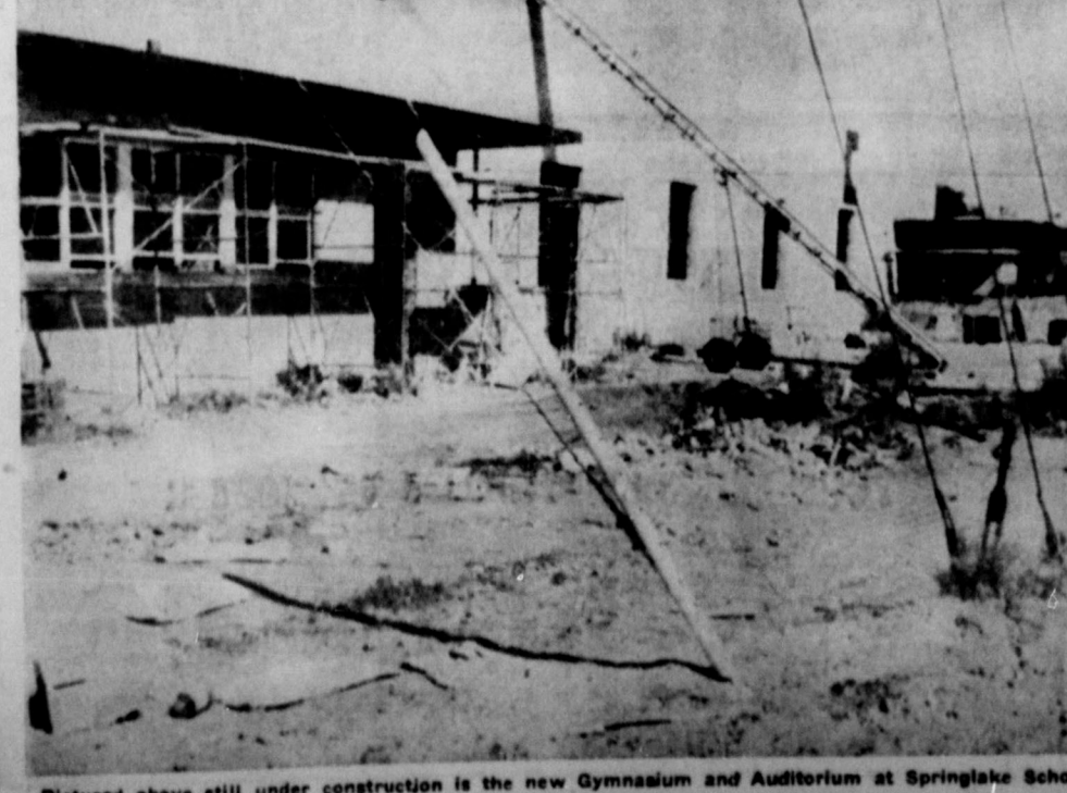
Pictured above still under construction is the new Gymnasium and Auditorium at Springlake School, next week.
