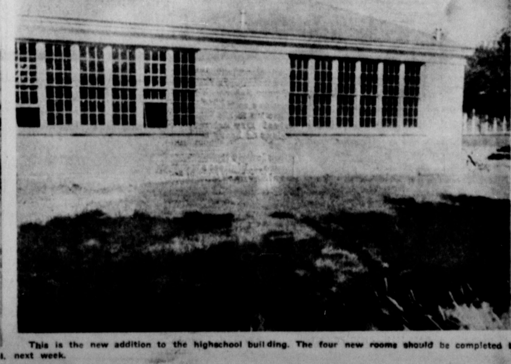
This is the new addition to the high school building. The four new rooms should be completed by next week.
