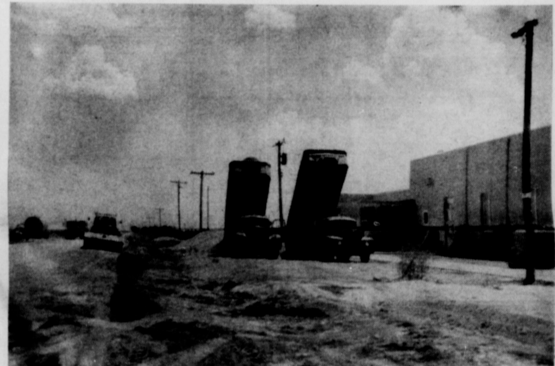
PAVING PROJECT — Gets underway at Springlake Schools. Drives, parking area, football entrance and road to bus barn is being paved. Also the State Highway Department is widening the highway directly in front of the schools. (Photo By Polly Jean Middleton)
