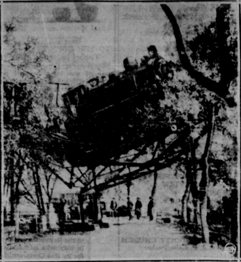
The dramatic critics who bemoan the lack of sustained suspense in lightly regarded shows they review ought to have been present at Dresden, Germany, while the locomotive hung precariously above the roadway. The bridge sagged when the locomotive crossed it, but fortunately for the many persons in the coaches, the steel structure didn't break, so no one was killed.
