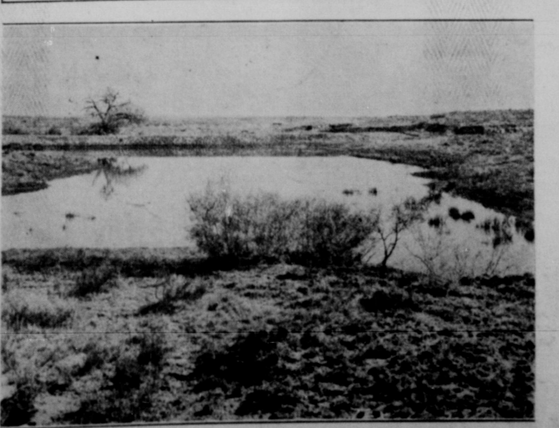
Above is shown the stock-water tank and dam constructed on the L. G. Yarbrough farm in Collingsworth County by Memphis Soil Conservation Service workmen. The tank drew wide interest when it was completed last September 3, as a heavy rain fell that night and filled the tank with over 3,000,000 gallons of water to relieve Mr. Yarbrough of his water-hauling duties.
