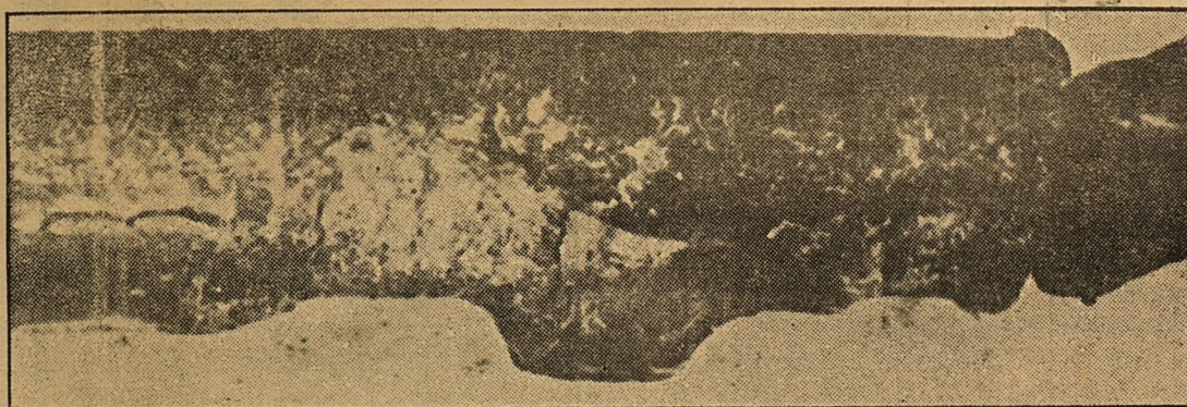
Above: Wire with insulation blistered. Such heating causes energy losses of as much as 25 per cent of light bulb or electric appliance efficiency.
