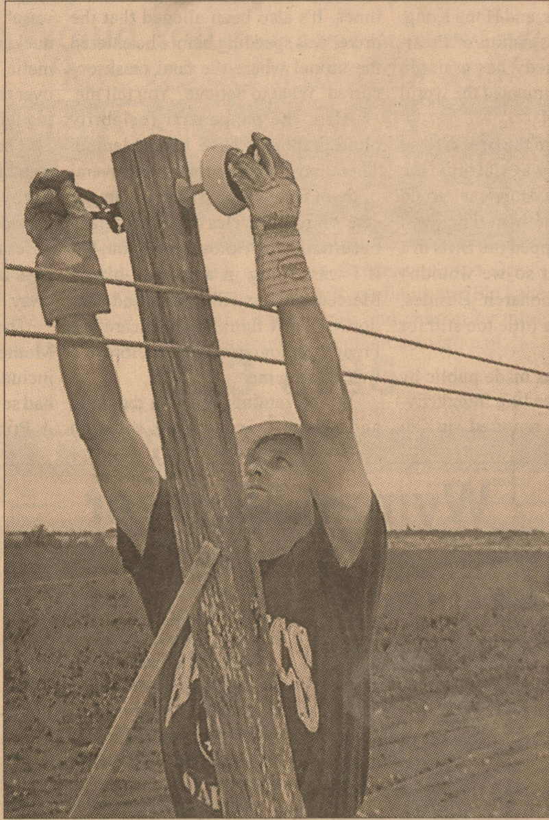
photo by Kathy Mankin All in a day's work — Dobs Lively works to clear downed power lines along US 190 East near the Eldorado Cemetery. Four poles belonging to Southwest Texas Electric Cooperative were snapped in a violent windstorm on Wednesday, August 3rd blocking traffic briefly. See related photos Page 10
