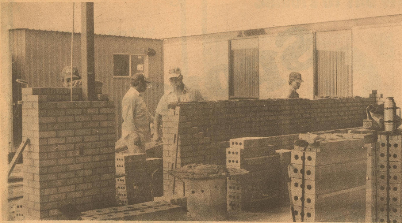
FINISHING TOUCHES--Workmen put up layers of bricks on what will be the business office and lobby for the nursing home when the new wing at Schleicher County Medical Center will be completed. Construction on the new wing continues daily. The project is expected to be completed sometime this summer. It will contain offices for three doctors. (Photo by Matthew Nixon)
