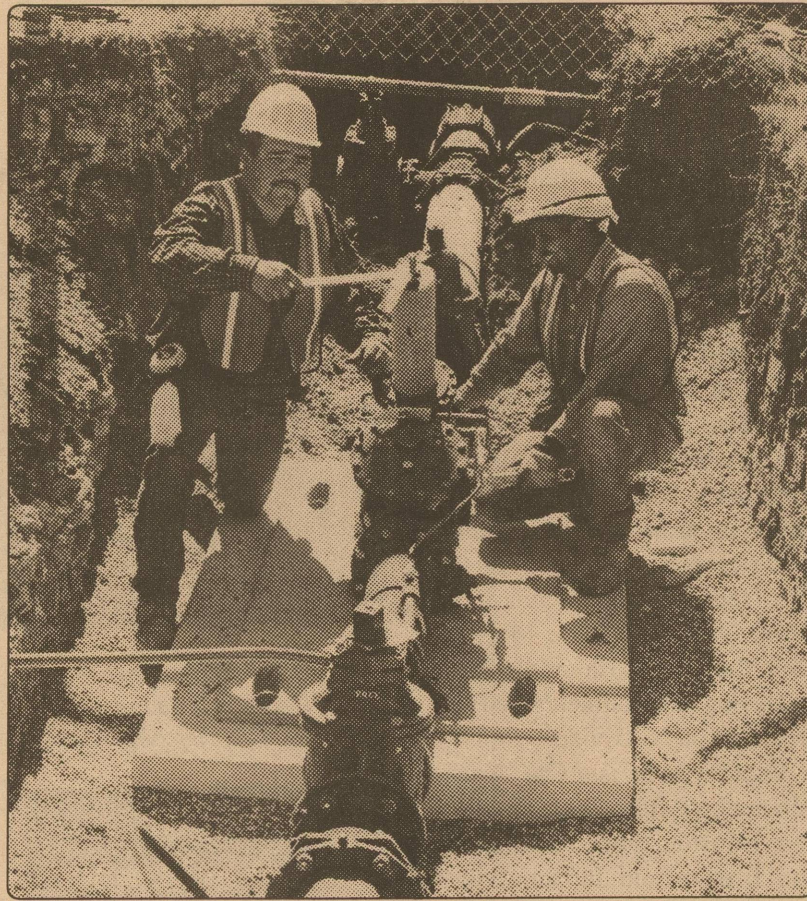
Down in the hole — Roberts Construction employees Greg Macias (L) and Paul Blanco (R) put the finishing touches on an "altitude valve" installed beneath the water tower behind City Hall. A concrete vault was placed over the valve, which was installed for the purpose of forcing the north water tower to fill, thereby increasing water pressure in on the north side of town.
