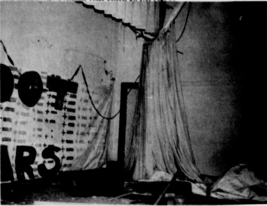
A BOLT OF lightning wrecked the stage at McLean High School last week, and caused damage to water lines at the school. (Photo by Linda Haynes)
