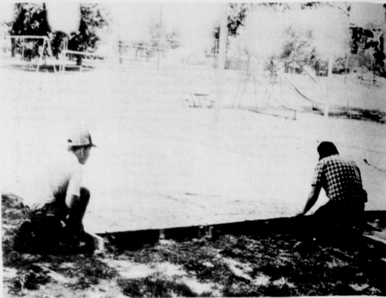
THE CITY PARK will soon have another concrete slab basketball court, as Trevor McDonald, left, and Jim Barker prepare the area to pour concrete. City officials said that the other slab had been so popular, they
