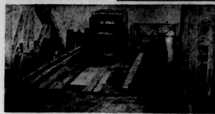
FIRST ACROSS... A U. S. Army vehicle crosses a 120 foot Bailey bridge constructed by engineers near Balgon, The Bailey span was built across an existing bridge that had been declared unsafe.
