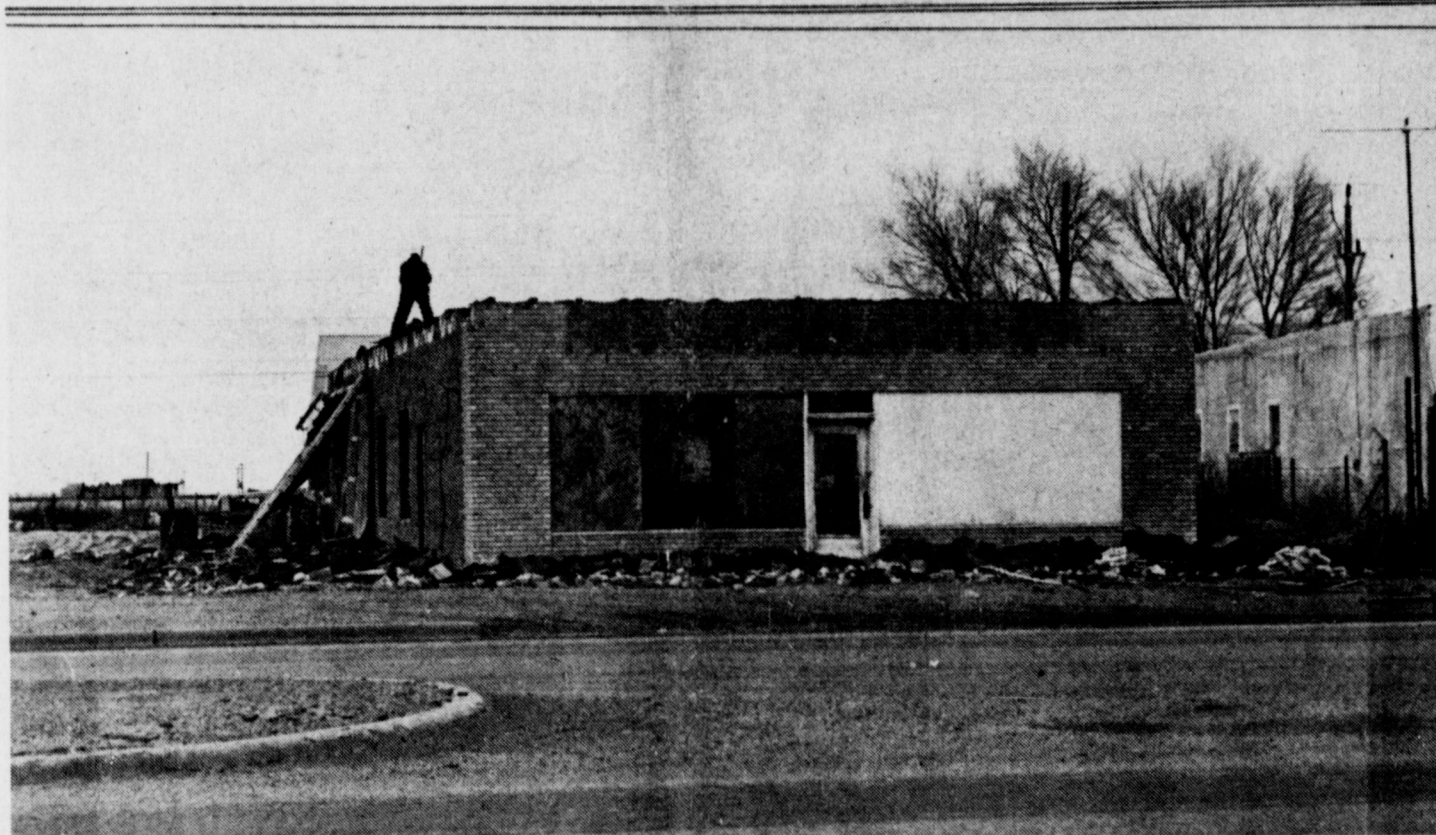
CONSTRUCTION TO BEGIN-- Demolition of a building on West American Blvd. is currently underway to make way for the construction of a new building which will house the Muleshoe branch of A&M Farm Supply, headquartered in Clovis. The new building is expected to be completed in the spring of 1980, and it will be operated by Weldon Stevenson, a Muleshoe resident, currently working in the A&M store in Clovis. It is the major construction planned for Muleshoe at this time.
