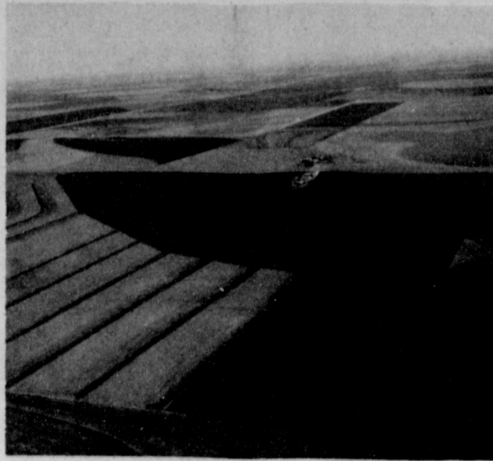
SOIL CONSERVATION PROJECT . . . Approximately 400 miles of parallel terraces have been constructed in Bailey County with assistance through the Great Plains Conservation Program. Pictured here are some of the terracing processes used.
