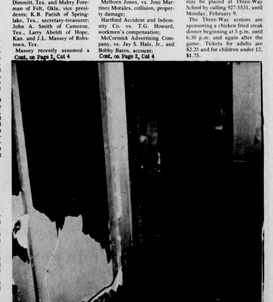
SPANISH BAPTIST CHURCH BURNS . . . Wiring in the ceiling caused a fire which completely destroyed the inside of the old building at the Spanish Baptist Church Thursday evening. The sanctuary only suffered smoke damage. H.E. Reeder, Muleshoe Fire Chief said this was the 25th fire during the month of January and the 29th since the first of the year in Muleshoe.
