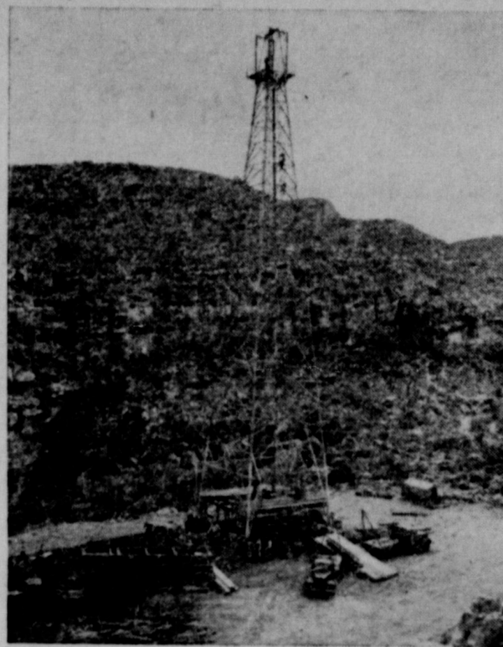
How to plan a wildcat. Planning kept this remote wildcat of a Humble Oil & Refining Company, on schedule. The well site is 30 miles southwest of Carlsbad, N. M., deep in the Guadalupe Mountains in the rocky depths of Last Chance Canyon. As the derrick nears completion, oil well machinery moves in to be set up for drilling.
